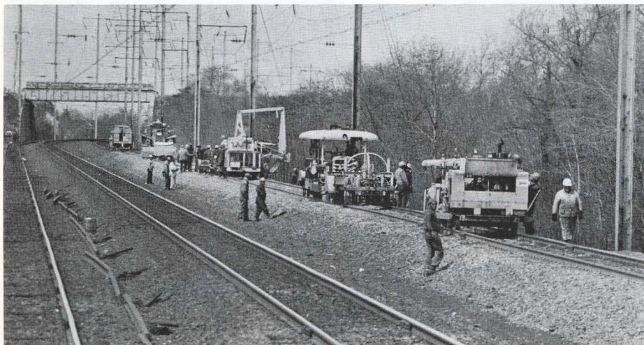
Track machines, strung out in a line near Odenton, Maryland, continue to work upgrading track for future 120-mile-per-hour train speeds.
